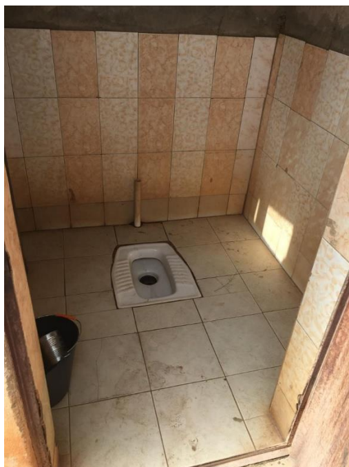
The third old toilet has no water supply
