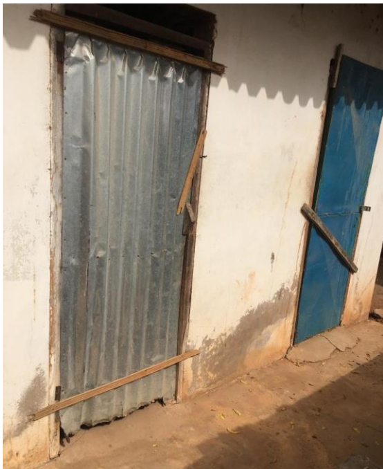
Two old toilets are out of action
