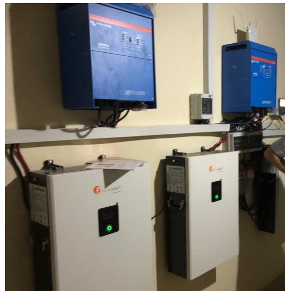
New solar power equipment
